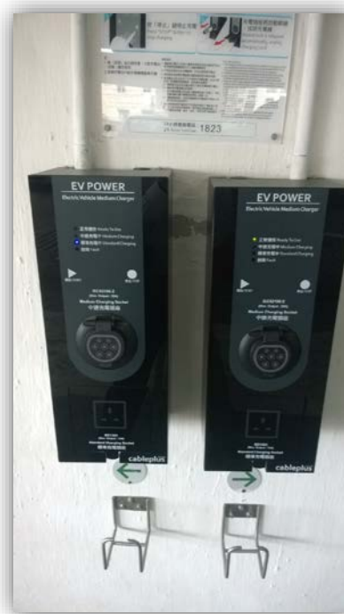
Figure 4-10 Semi-quick EVSE in Hong Kong
