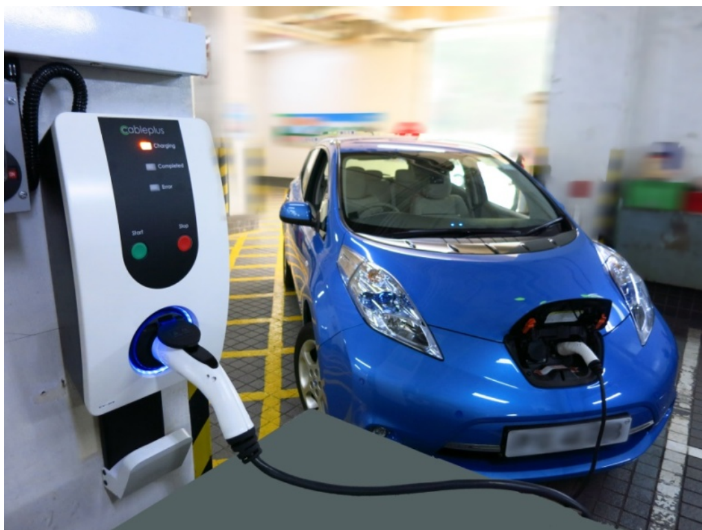
Figure 4-3 Semi-Quick charging EVSE
