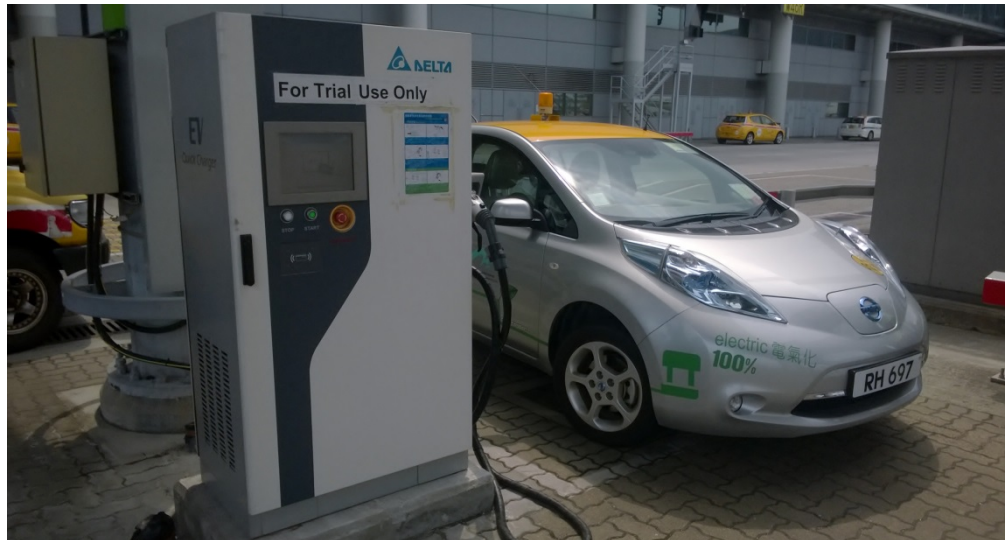
Figure 4-4 DC Quick charging EVSE
